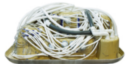
Spa-ghetti? The spa above shows how a traditional "Me-Too" hot tub is plumbed
